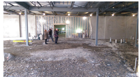
Fr. Bob and Debbie Lestarczyk are standing in what will be the main hallway/lobby.
