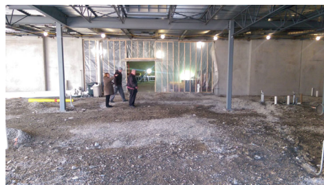
Fr. Bob and Debbie Lestarczyk are standing in what will be the main hallway/lobby
